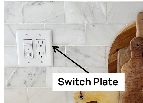
Flat Tile with electrical box: No gaps
